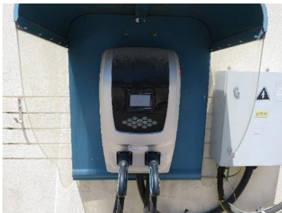
80 kW, 3-phase AC quick charging facility
