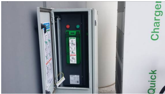
Charging facilities (installed within airport by Airport Authority Hong Kong)
