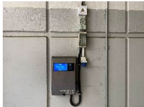
The Charging Facility 2
