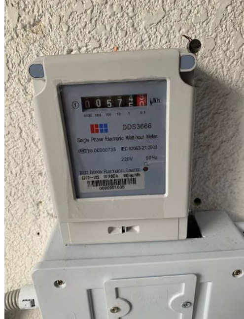
EV – watt-hour meter
