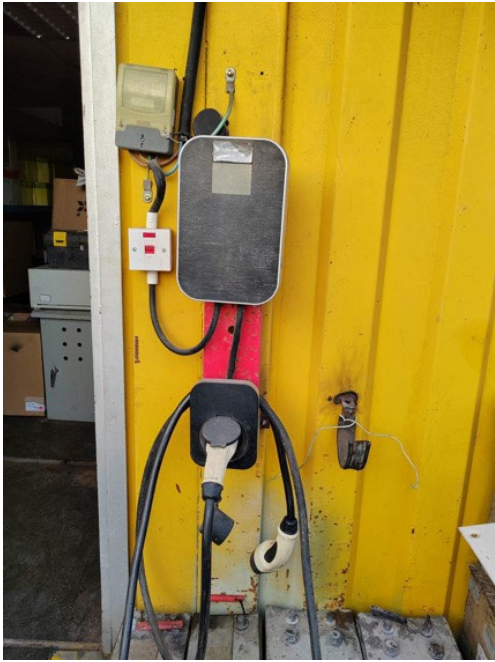
The charger and the electricity meter
