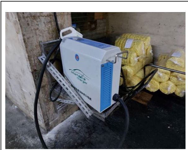
30kW DC charging facility
