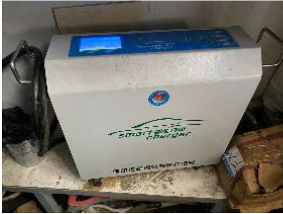
30kW DC charging facility
