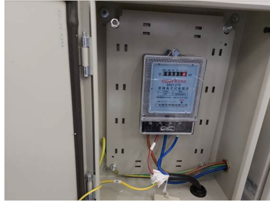
EV – watt-hour meter
