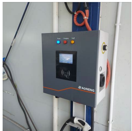
22 kW AC charging facility
