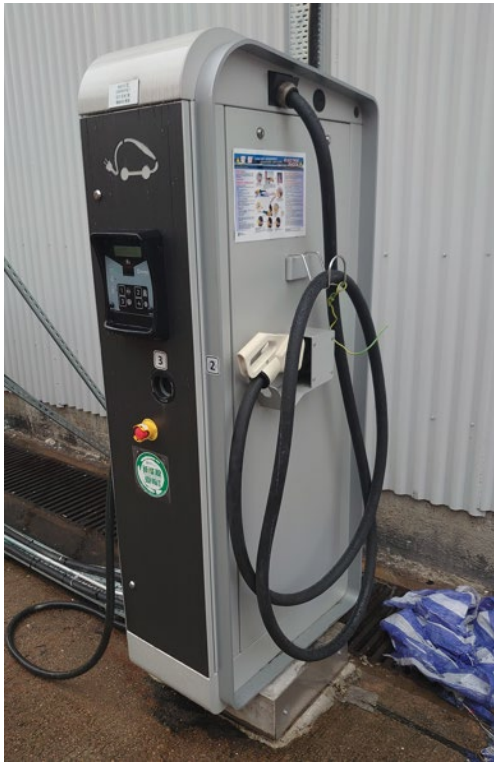
Charging facility – 50 kW DC quick charger in Container Terminal 2
