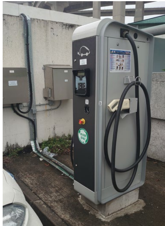
Charging facility – 50 kW DC quick charger in Container Terminal 9 (South)
