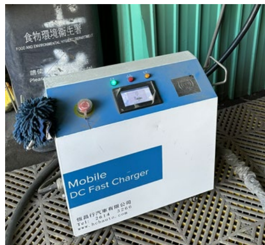
30 kW DC Charging Facility #2
