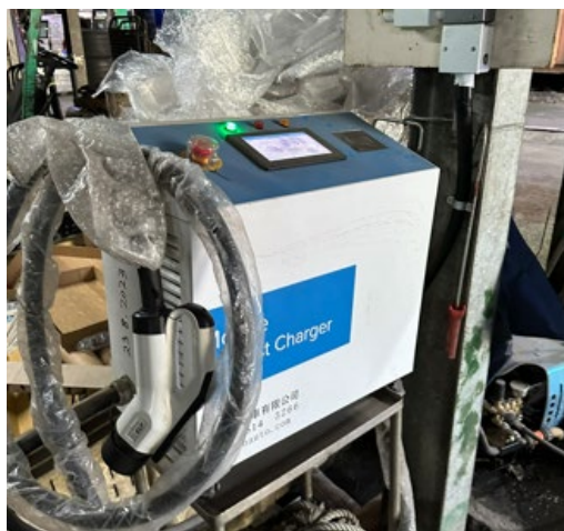
30 kW DC Charging Facility #1
