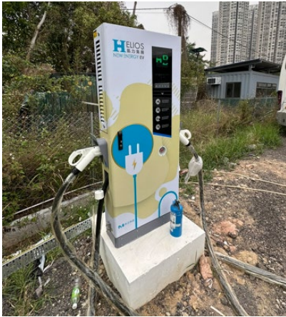
60 kW DC charger at Tin Shui Wai (at Recipient's own cost)
