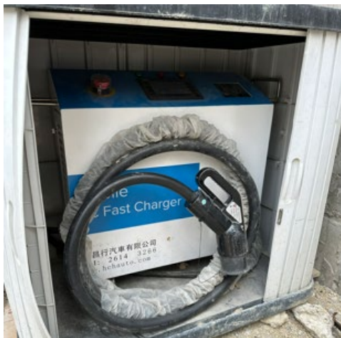
30 kW DC charger #3 at Hin Fat Lane construction site, Tuen Mun
