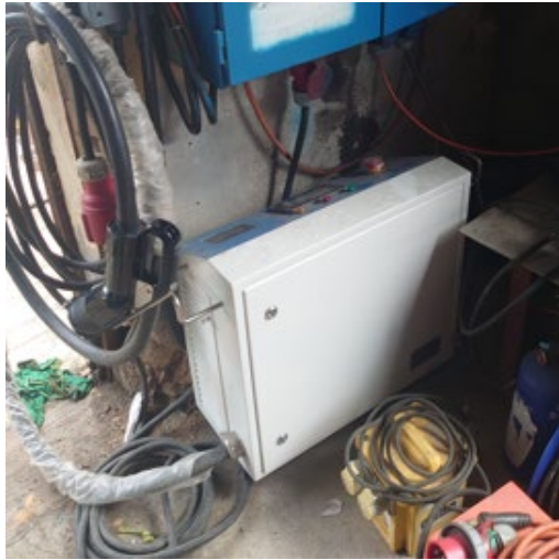
30 kW DC charger #1 at Ping Che warehouse
