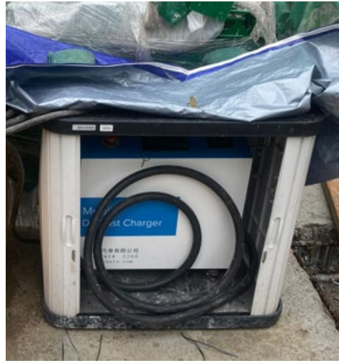
30 kW DC charger #2 at Muk On Street construction site, Kai Tak
