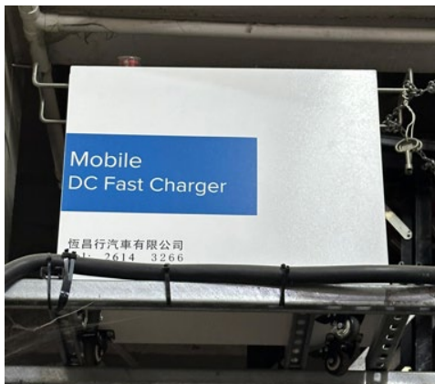
30 kW DC Charging Facility #1
