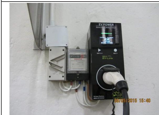
EV charging station
