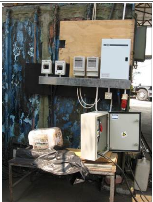
Charging facilities at Chi Shing's office in Yuen Long
