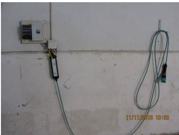
EV Charging Station
