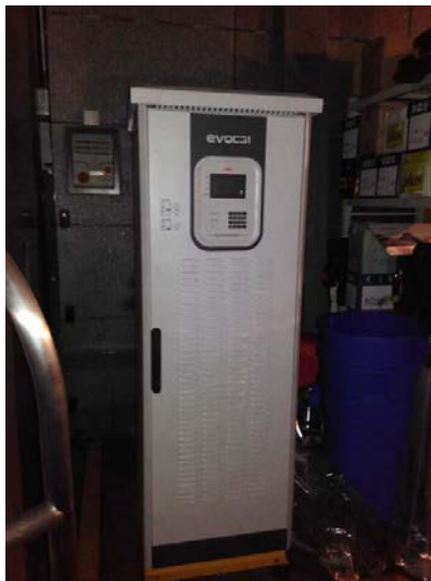
AC/DC converter installed in baggage room on ground floor (serve charger at ground floor)
