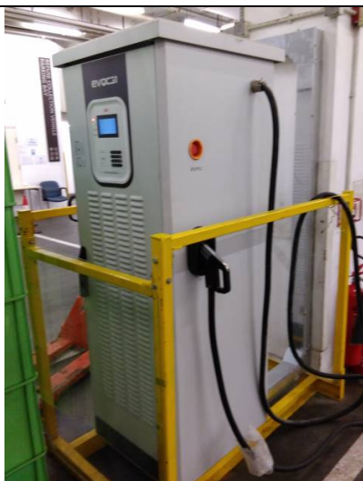
Complete set battery charger installed in basement floor for charging the EVs
