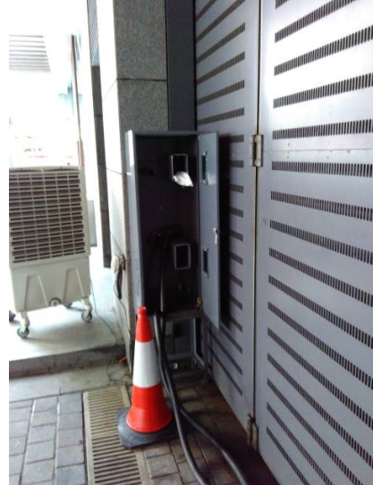
Battery charger (with charging cable) installed at ground floor
