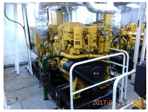
#2 main diesel generator (for propulsion)
