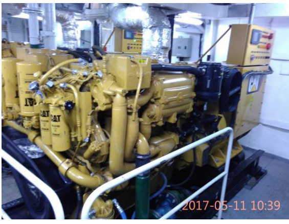
#1 main diesel generator (for propulsion)
