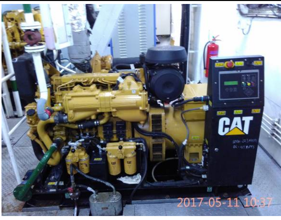
Auxiliary diesel generator
