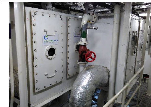
Seawater Scrubbers with exhaust inlet
