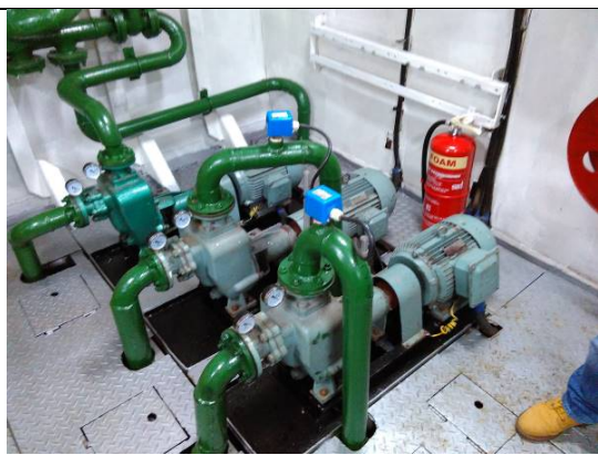
Seawater pumps for seawater scrubbers
