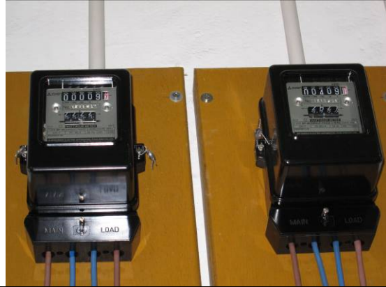
Watt-hour meters at charging station
