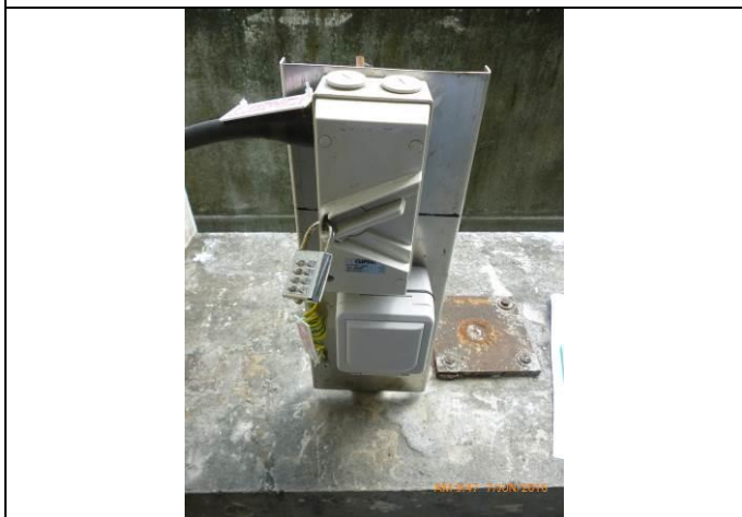
EV Charging Station
