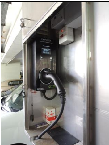
EV charging station
