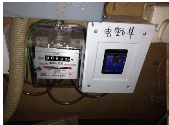
Watt-hour meter for the charger
