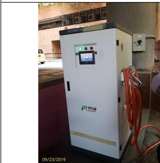
Charging Station 80A
