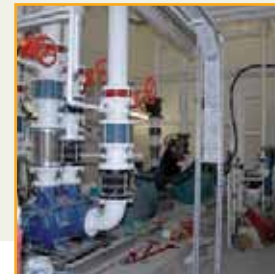
Sprinkler fixed & fire services booster pump room
