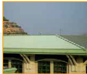
Non-absorbing roofing – roof covered by light-coloured or reflective membranes - absorbs less heat
